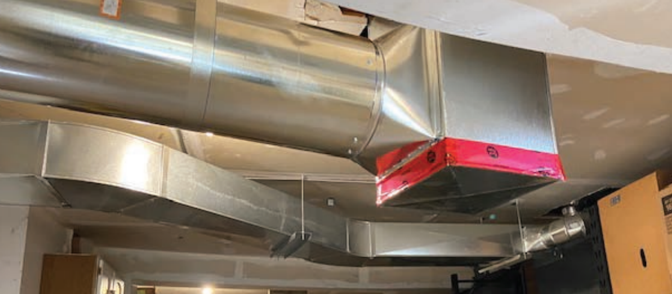
New heat pump ventilation system at St. George and St. Andrew United Church.
