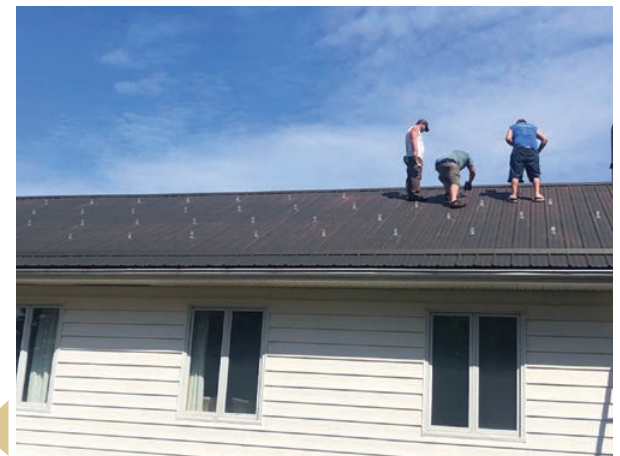
Workers installing solar panel system on the roof of Old Barns United Church.
